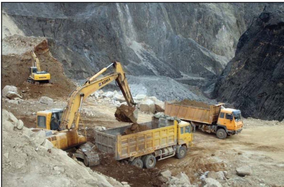
Excavators dig rare earths at Jiangxi Copper Corp’s Sichuan branch in Chengdu, Sichuan Province of China. (ChinaFotoPress)
